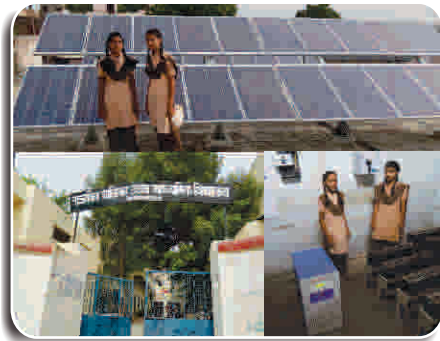
5 KWp SPV Power plant installed at government senior secondary school, under PSU CSR initiatives
